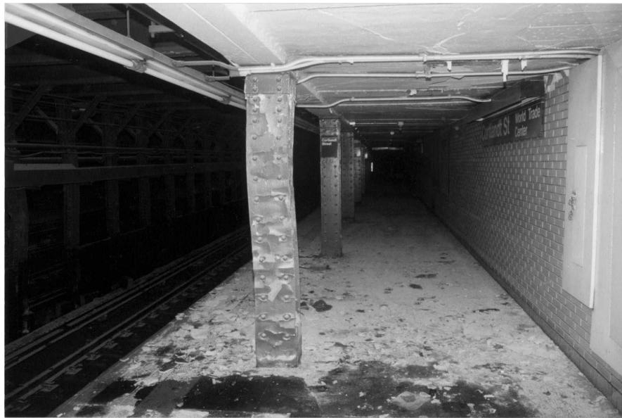
Figure 10.2. Impact buckling of a steel support column in Cortland St./WTC Station (New York City) after the collapse of the World Trade Center on Sept. 11, 2001. Photo by MTA New York City Transit. Permission to be obtained.
